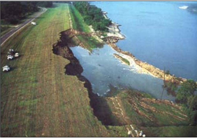
Levees can fail for many reasons. Above: An unexpected levee break in California's central valley in 2004 caused $90 million in damages; exact cause is unknown but poor maintenance may have been an issue. (Photo: Calif. Dept. of Water) Below: A massive slope failure in Louisiana in 1983.
