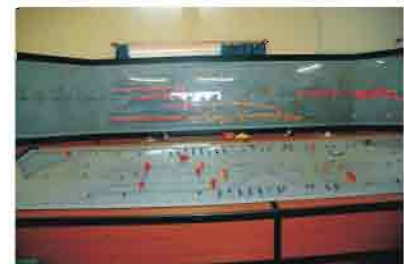
Route Relay Interlocking system at Bandra Terminus, Western Railway.
