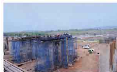
View of a bridge construction work in Western Corridor - Pier cap in river Sanjan, (DFCCIL).
