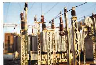
54 MVA traction transformer for 2x25 KV TSS.
