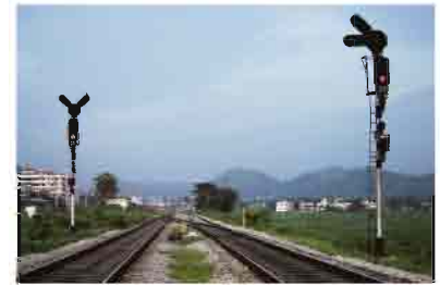
LED Signal, Northeast Frontier Railway.
