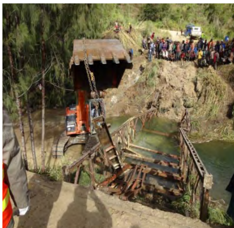
A collapsed bridge on the Mendi–Kandep road, Southern Highlands Province, July 2013.
