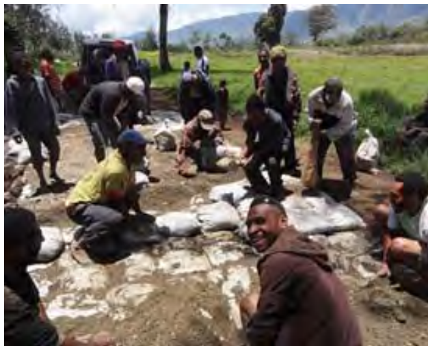
Villagers quickly master the do-nou method of rebuilding and maintaining rural roads.
