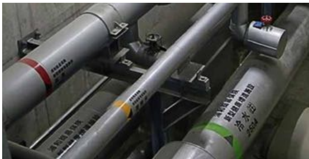
Separate piping system for water supply and treated wastewater.
