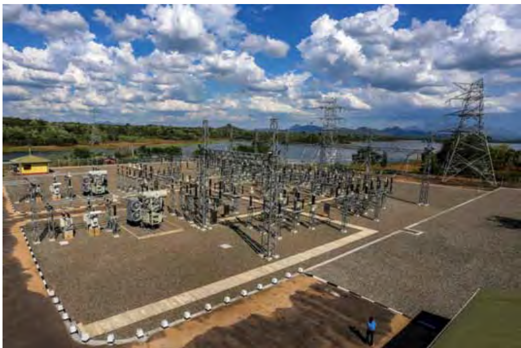
The switchyard of Mahiyanganaya Grid Substation at Dambarawa- Mahiyanganaya
