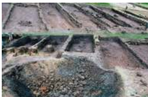
Works to renovate tank and excavation of silt, Mogullapally mandal, Warangal, APMSS
