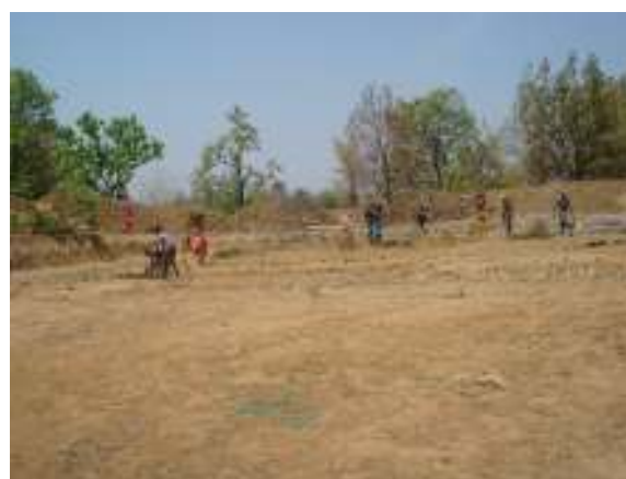
Work under progress on a WHS site in Nuapada, facilitated by Lokadrusti
