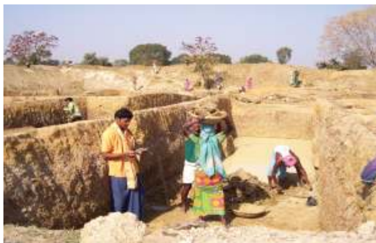
Work in progress at Muribahal under MGNREGA to construct a water harvesting structure
