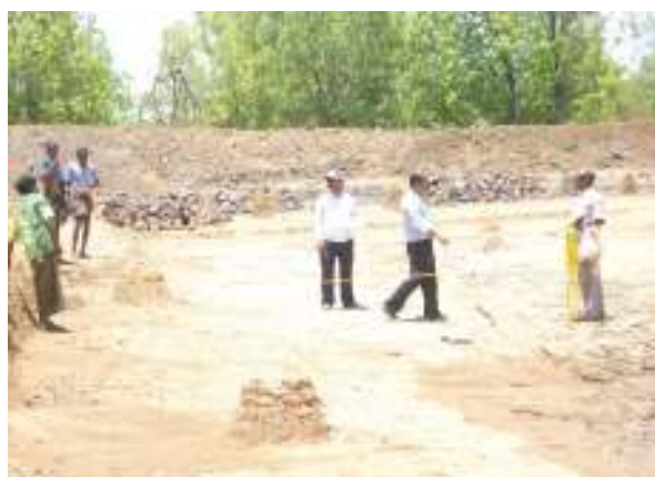
Construction of a water harvesting structure at Sunapur in Boden block, Nuapada, a Lokadrusti operating area
