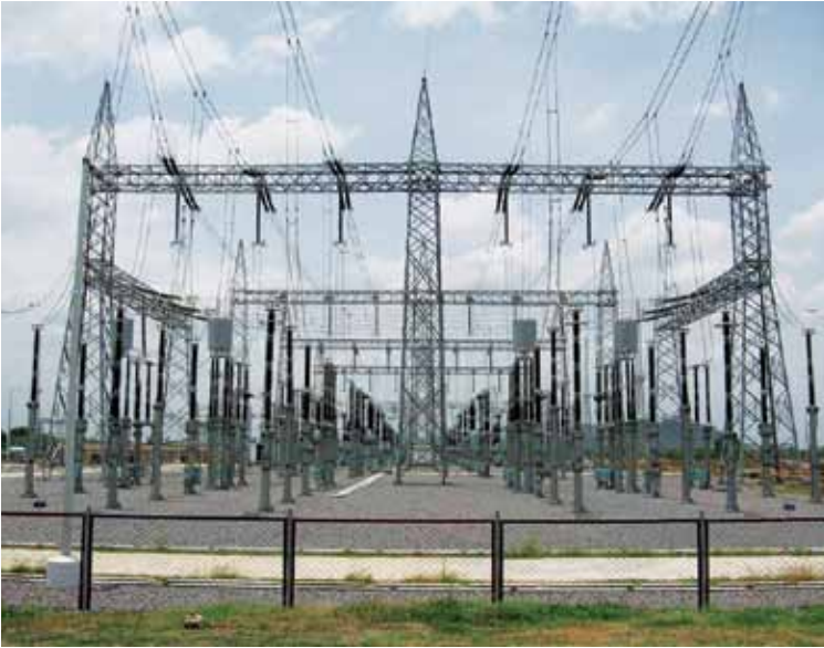
ADB-supported power grid in Warangal
