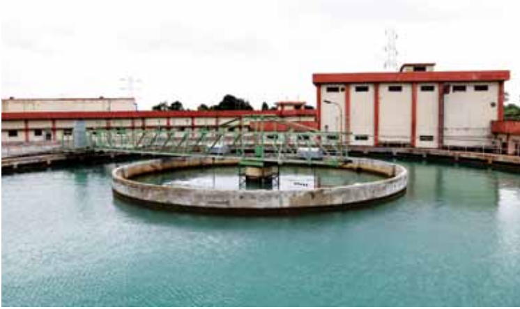
Water treatment plant constructed under UWSEIP, Jabalpur
